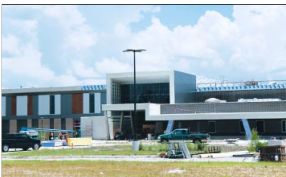
North Forest High School's new building while it was under construction. Recently, the transition to the new renovated building took place on Mesa Road.
