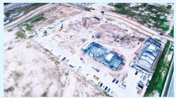
Drone photo in October showed road construction, and BakerRipley buildings framed out.
