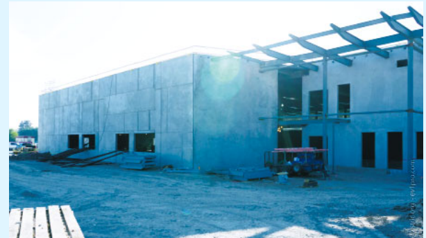
Harris County 9-1-1 Call Center is built of concrete to withstand Force 5 Hurricanes and still function.
