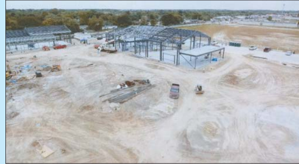
Drone Aerial photo showing BakerRipley structural steel, and roadwork through the site. (Drone photo courtesy EV 1 Productions).
