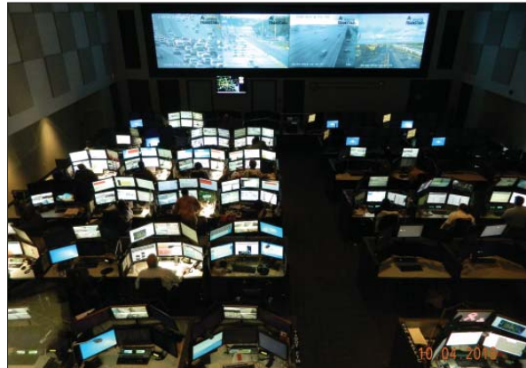
TranStar facility includes two control rooms. The one above is for normal traffic. On the left are monitors and operators for the Metro bus system, and the light rail network. On the right, are operators controlling the traffic signs throughout the greater Houston area, and in the lower right are dispatchers to help in emergencies or traffic jams.
