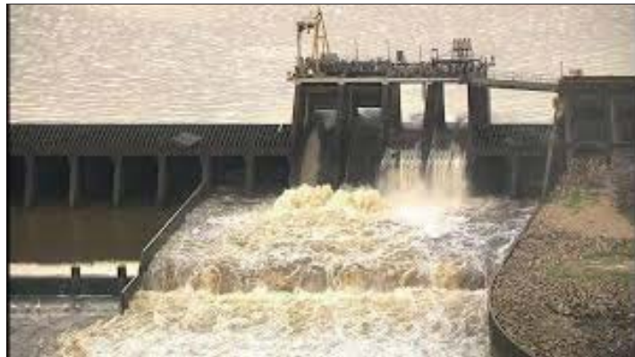
The existing flood gates consist of two radial gates used to release high volumes of water and two flashboard gates to accurately affect water levels on Lake Houston.
