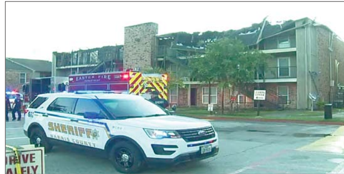
EARLY MORNING HOURS on Friday show the extent of the damage to the building at Haverstock Hills Apartments. The top floor and roof of the building are completely destroyed, and lower floors have some smoke and water damage. The building is uninhabitable and will need to be taken down.
