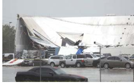
Three workers were injured when part of the roof of the Post Office on Aldine Bender collapsed.
