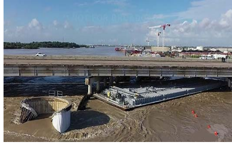
Nine barges broke loose from moorings due to high water, and damaged the I-10 bridge over the San Jacinto River, causing TxDot to close all traffic.
