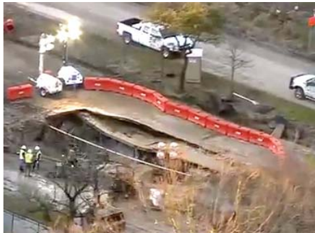
BROKEN PIPE IS UNDER REPAIR ALONG CLINTON DRIVE.
