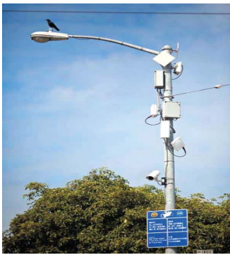
Shotspotter equipment pole mounted
