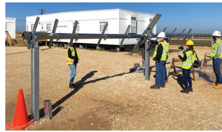
Lone Star College and RigUp have teamed up to provide free training for students interested in joining the growing renewable energy industry. Pictured are solar professionals constructing a solar farm at Round Rock, Texas.
