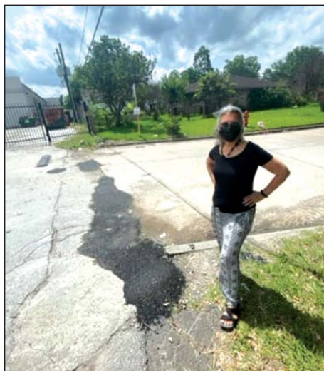
Marina Sugg of the Green Forest CCivic club inspects a Pct. 2 Pothole Repair in the East Aldine area.
