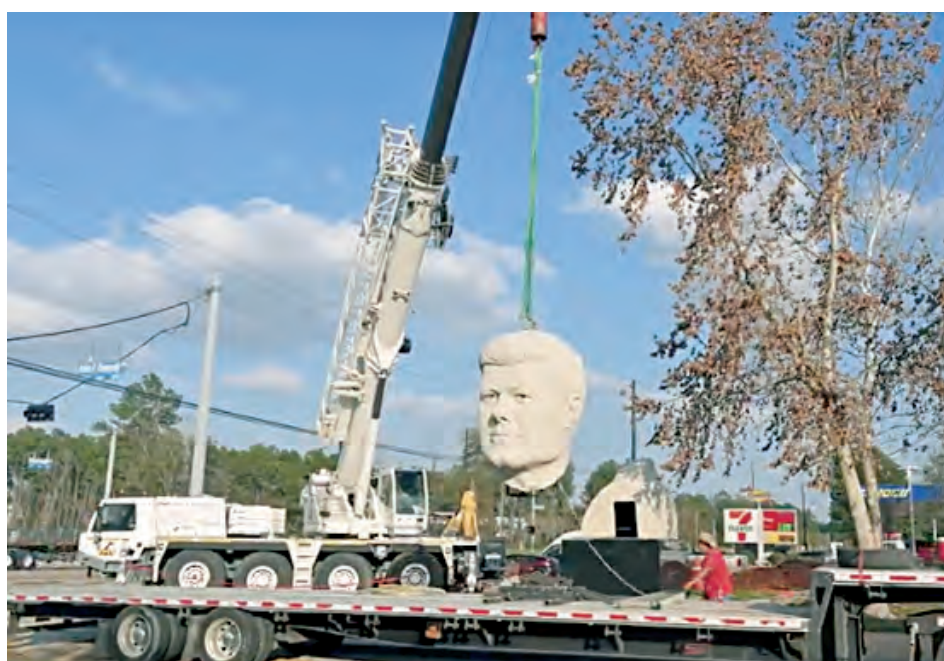
Workmen carefully lift the head of the JFK sculpture onto the base, which already has the torso in place (see photo, page 2). The sculpture was built in Adickes’ workshop in downtown Houston prior to installation in East Aldine.
