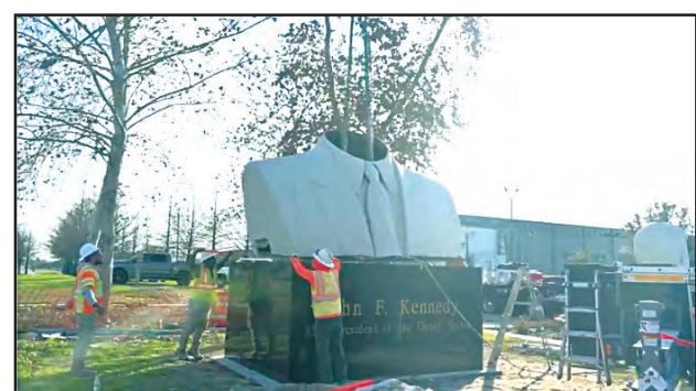
The JFK memorial sculpture is in three parts. Above, workmen affix the torso to the polished granite base, preparing for the placement of the concrete head on top of the torso and base.
