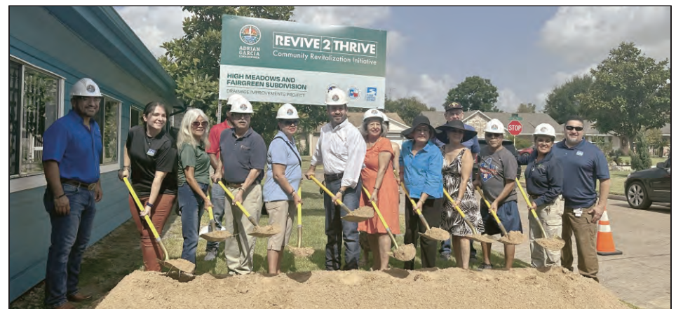
GROUNDBREAKING for the High Meadows & Fairgreen Subdivision Drainage Project was held last Wednesday, July 26 at a site on Debeney Drive. Seen ABOVE at the Groundbreaking are Pct. 2 Commissioner Adrian Garcia and members of the Harris County Engineering Department, Flood Control District, Community Services Department, East Aldine Management District Staff and Board Members, and Community Residents.
