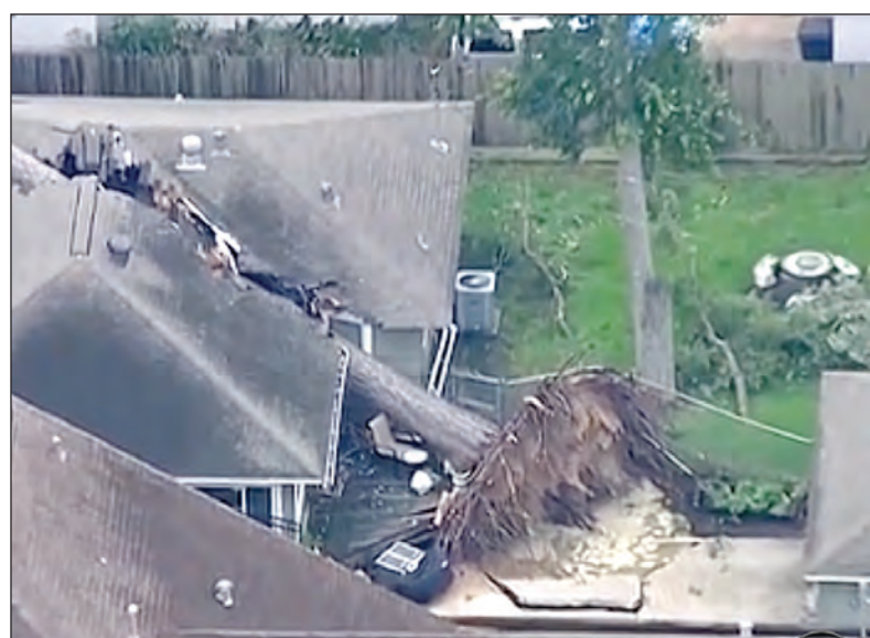
A tree uprooted from a backyard location, crushes the roof of a house in Houston.
