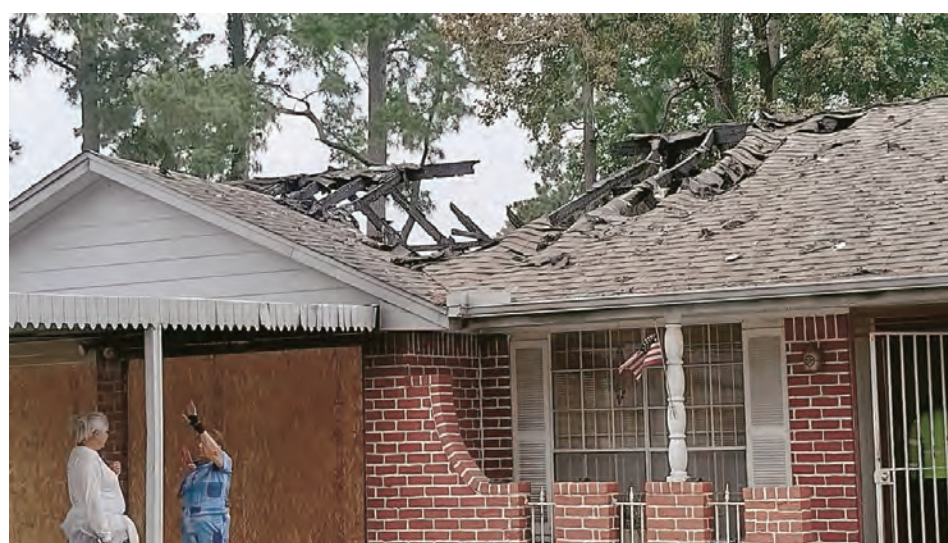
A VIEW OF THE ROOF AND HOUSE DAMAGE THE NEXT DAY.
