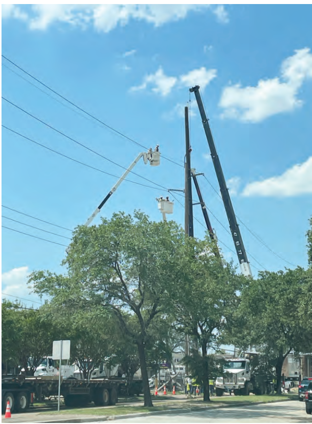
CENTERPOINT LINEMEN, HIGH IN THE SKY, REPLACE A POWER POLE. THIS OPERATION TOOK 12 TRUCKS, SPECIAL DRILLS AND CRANE, AND ABOUT 20 LINEMEN.
