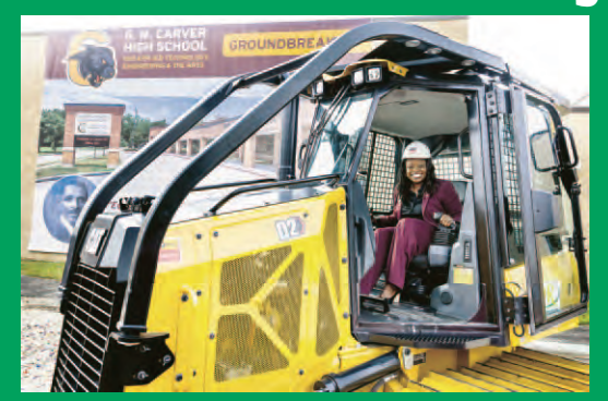
Aldine ISD Superintendent Dr. Goffney takes over the big shovel at the Groundbreaking. Story Below
